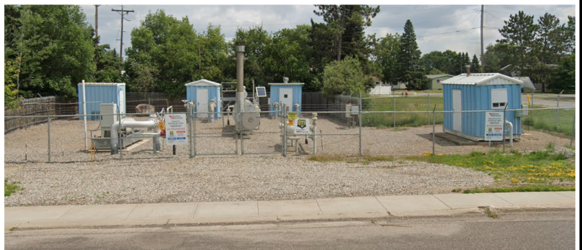
Town Border Station (TBS) located on Hwy 7 and feeds Virginia proper.
